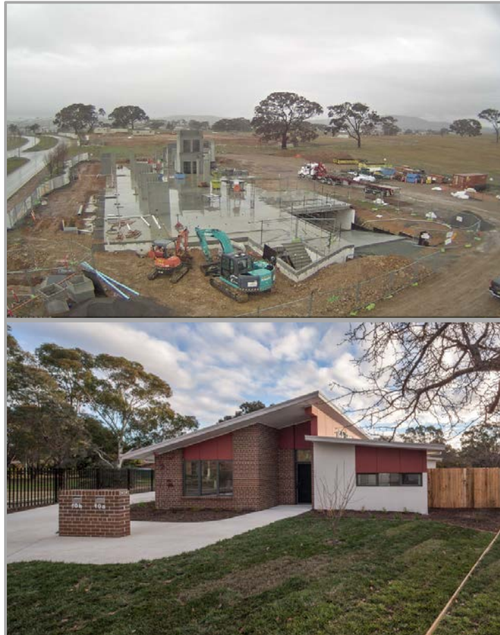
Top: Construction on Common Ground Housing at Gungahlin Bottom: Disability Dual Occupancy Housing at Richardson
