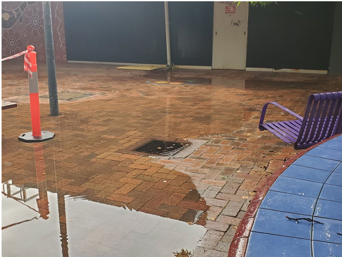
Dickson Shops after recent rain showing water backup from drain. Note pools cover nearly entire width of public space.
