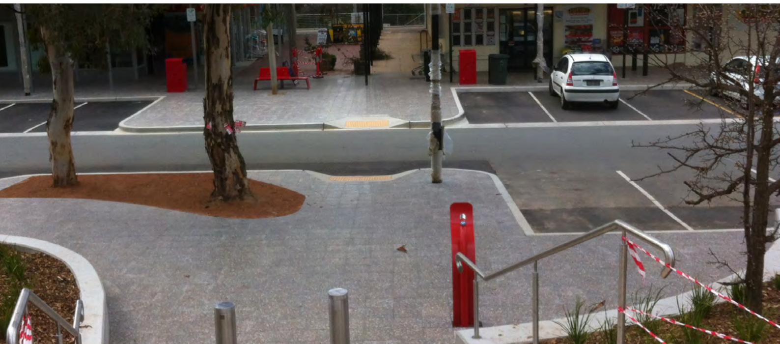
Paving and Stair Upgrades have been completed at Red Hill Shopping Centre
