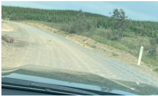
A deadly sloping road with no clear view of the dangerous curve ahead.
