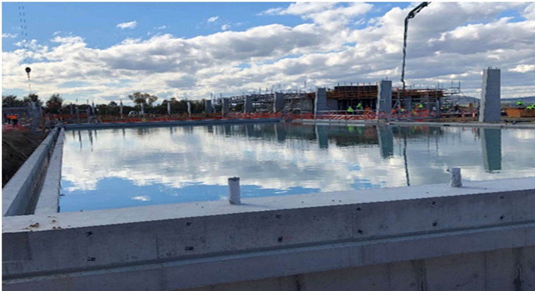
Stromlo leisure centre: The concrete structure of the 50 metre pool has been poured and water testing is currently underway
