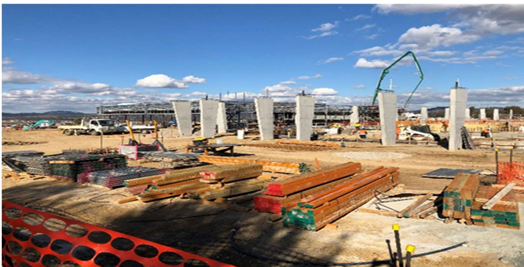
Stromlo leisure centre: Pouring of the concrete columns to the northern, southern and east pool hall are complete
