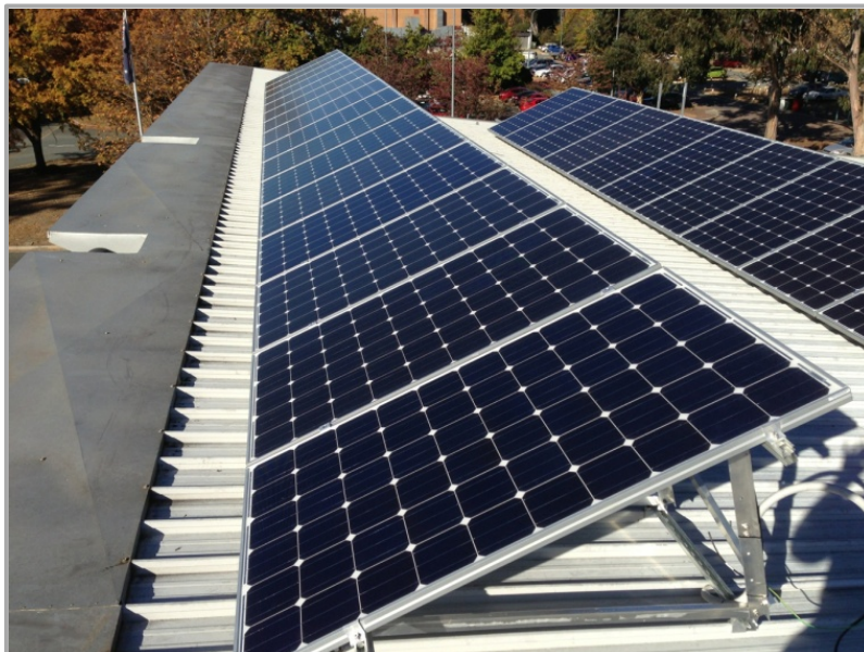
Capital Upgrades – Ainslie Fire Station Solar Panels
