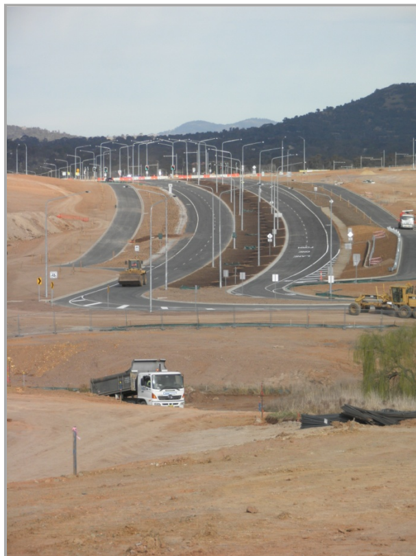
Stage 1D of John Gorton Drive Extension, looking back toward the completed section
