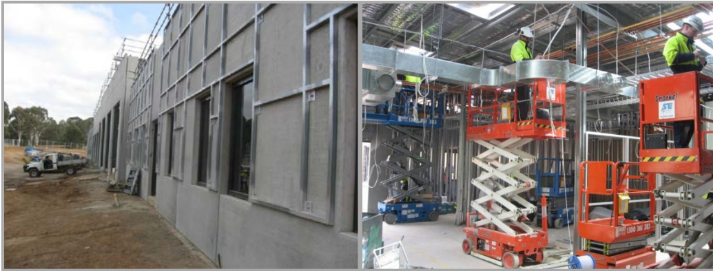
Left image: front facade of the ESA Station Upgrade and Relocation – Charnwood Station. Right image: Internal electrical fitout
