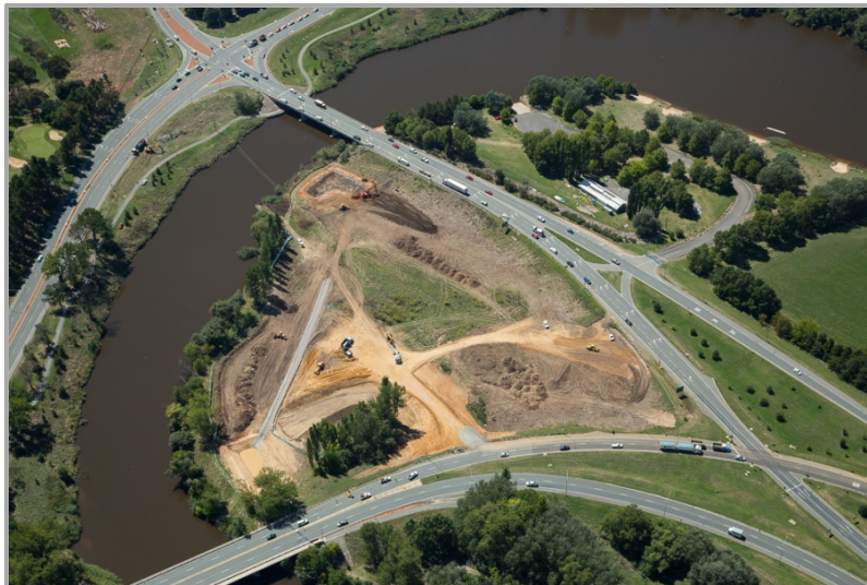
Aerial photograph of preparation for the construction of the new Molonglo River Bridge at the southern end of the Majura Parkway
