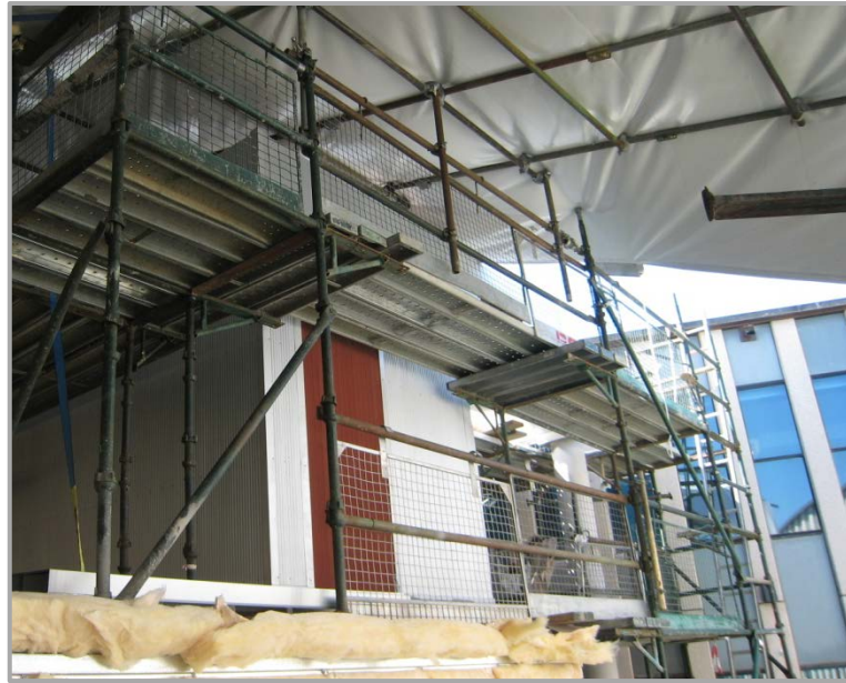
Replacement of the Chamber Roof and Facade at the Legislative Assembly Building
