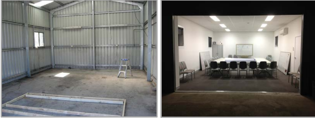
Left: Image of the shed before the refurbishment. Right: after the refurbishments the shed is now a fully equipped Training Room at Kambah Fire Station
