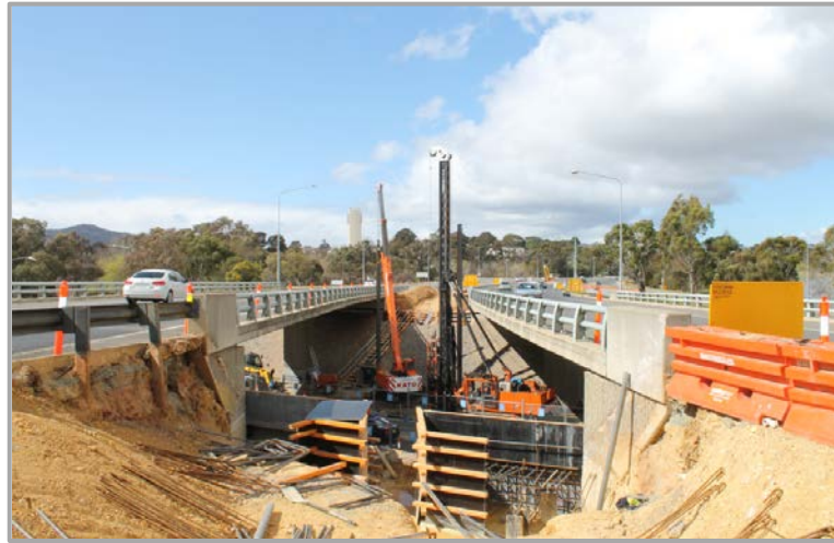
Construction of piers and pilings on the Parkes Way Bridge over Clunies Ross Street
