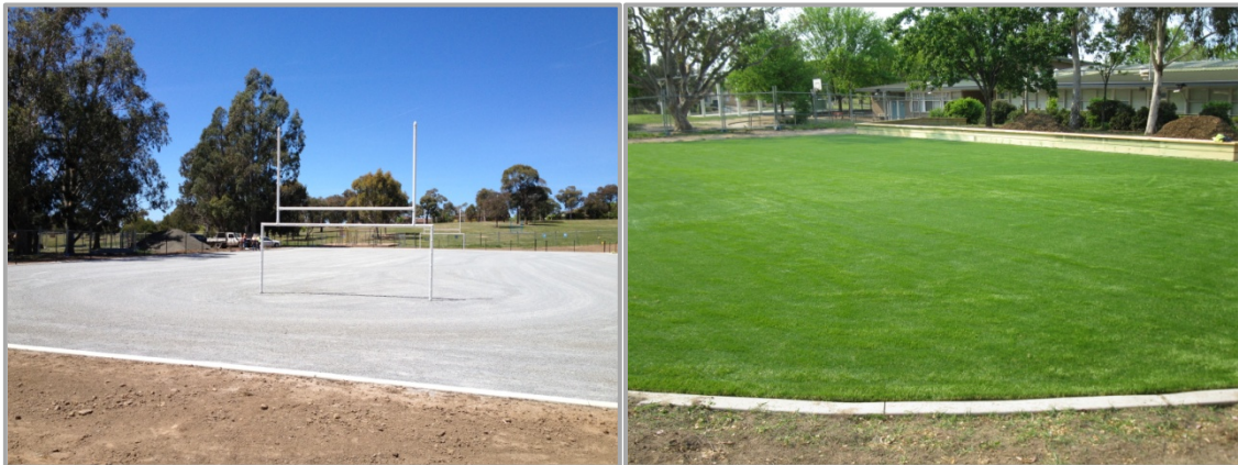
Left Image – surface preparation for installation of artificial grass Right Image – Completed artificial Grass Playing surfaces at Torrens Primary School
