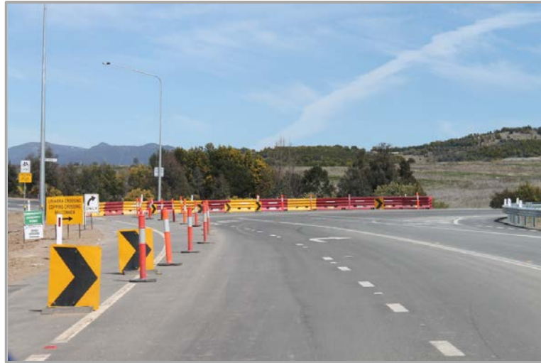
North-South Arterial Road for Molonglo Suburbs – Intersection of John Gorton Drive and Uriarra Road
