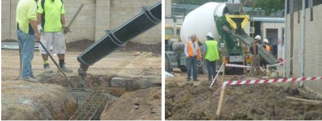
Concrete trenches and footings being poured at the New Forensic Medical Centre
