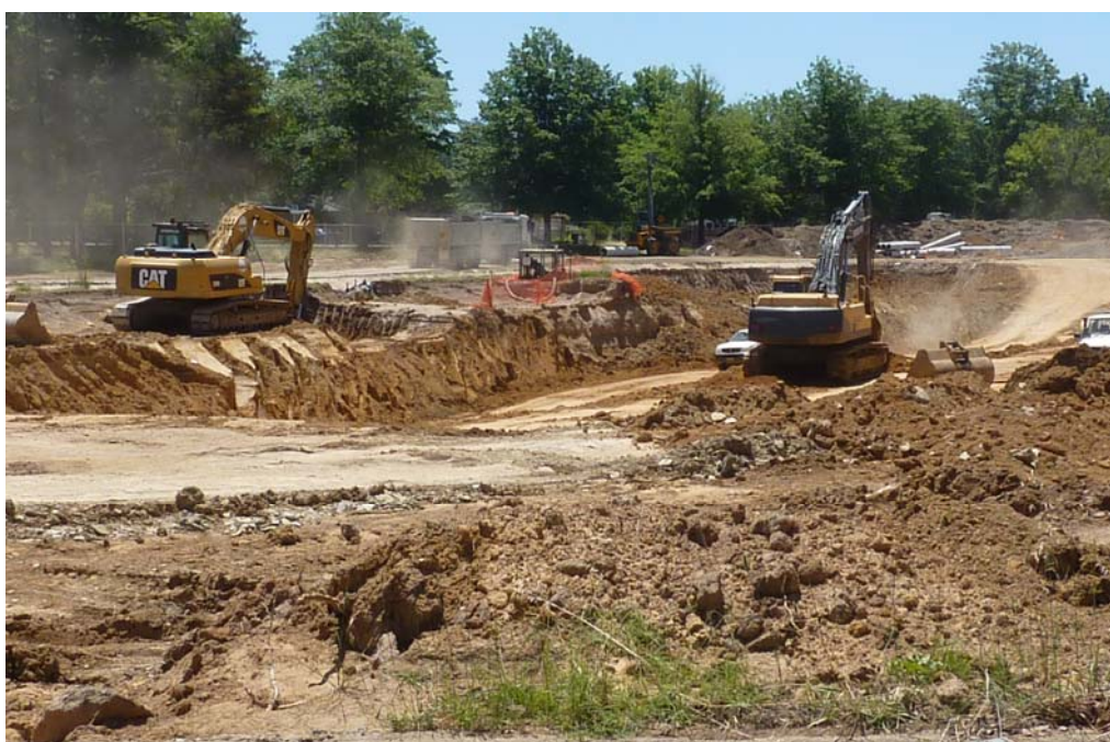
Works progressing on the new wetlands in Lyneham adjacent to Wattle Street
